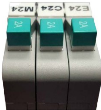
Figure 115: Breakers in the OFF Position
