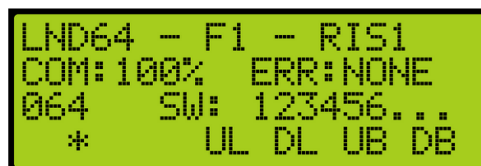
Figure 386: Hall Lantern Status for the 64 th Landing
