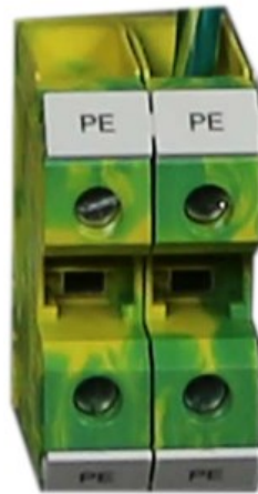
Figure 6: Ground Bus Terminal Blocks
