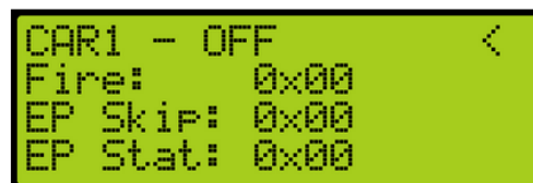
Figure 683: Fire Emergency Power Status Menu
