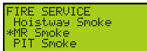
Figure 577: FIRE SERVICE Menu – MR Smoke
