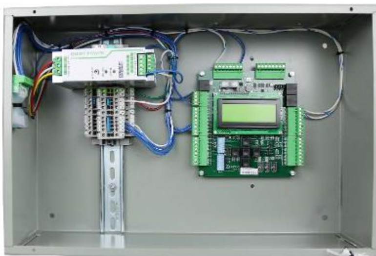
Figure 3: Car Top Controller
