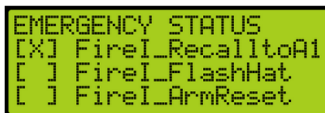
Figure 606: EMERGENCY STATUS Menu
