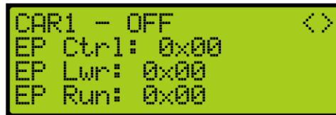
Figure 588: Emergency Power Status Menu
