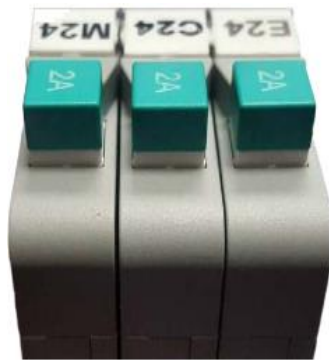
Figure 73: Breakers in the OFF Position
